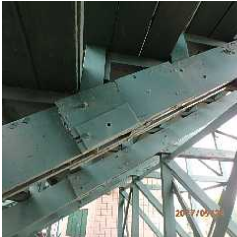
Photo 33: Structurally augmented stringer.
