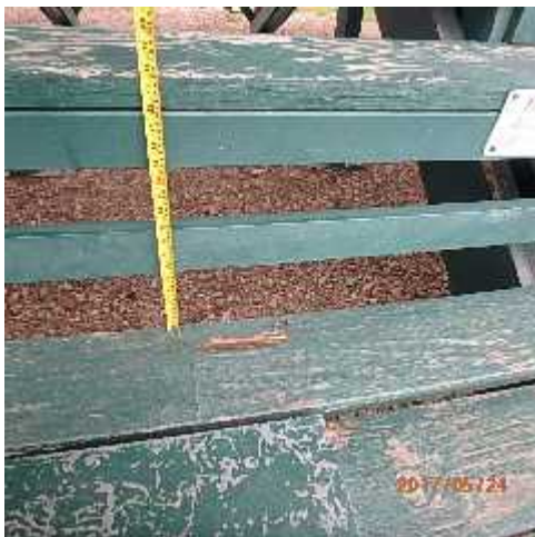
Photo 49: Typical gap between floor board and seat.
