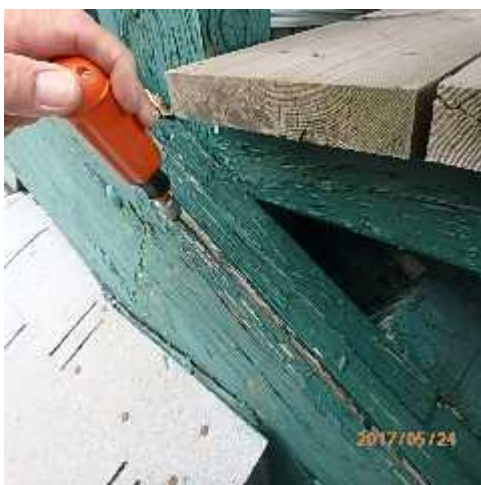
Photo 29: Typical wood deterioration.
