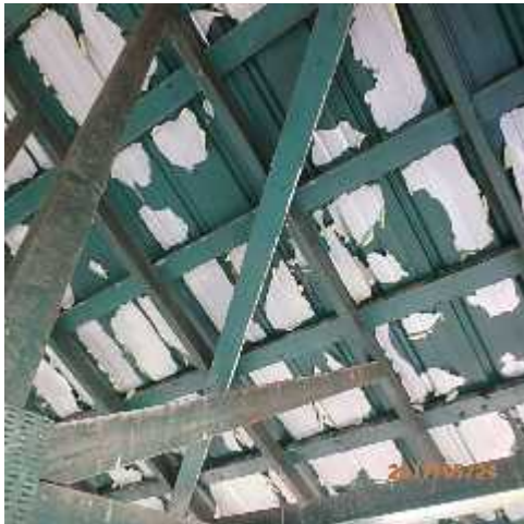
Photo 5: Peeling paint on underside of deck.
