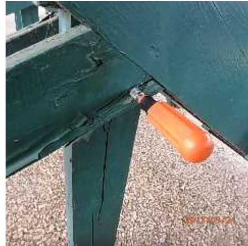
Photo 32: Wood rot at horizontal tie.
