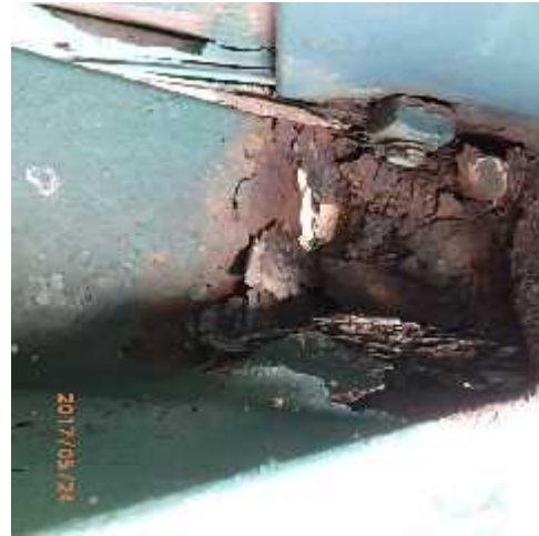
Photo 22: Typical steel corrosion.
