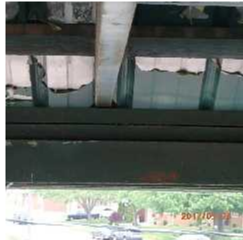
Photo 6: Peeling paint on underside of deck.
