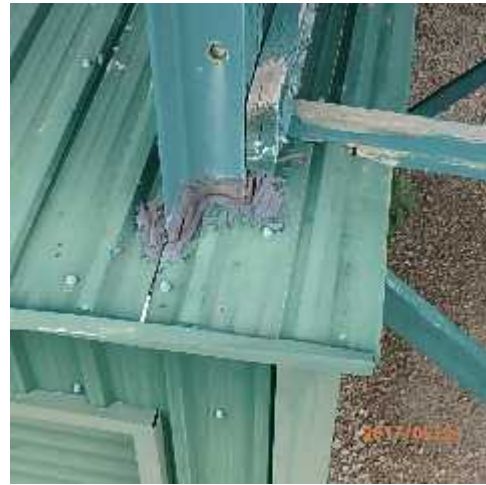
Photo 52: Poor waterproofing detail.
