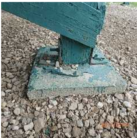
Photo 45: Typical post base deterioration.
