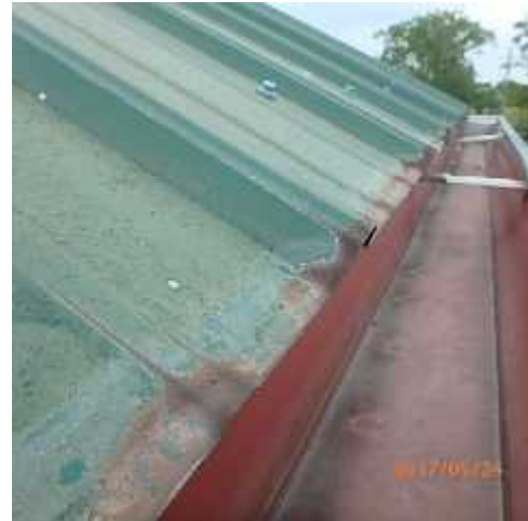
Photo 4: Paint erosion and minor corrosion.
