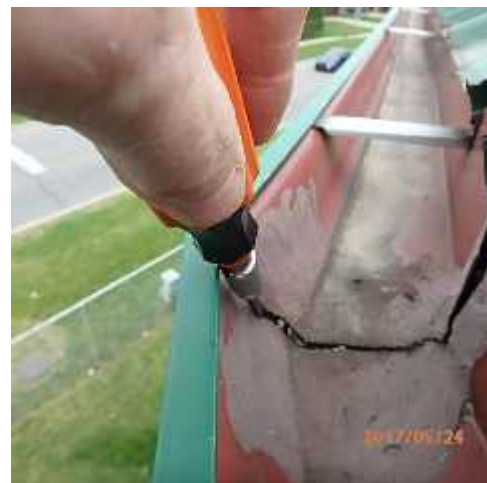
Photo 8: Eave trough separation.
