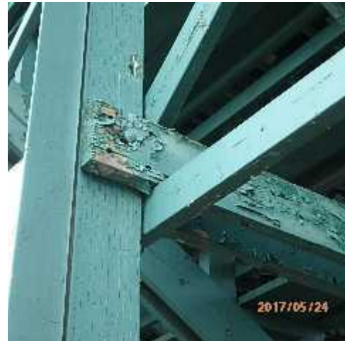
Photo 34: Typical paint and wood deterioration.
