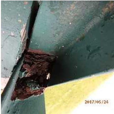
Photo 21: Steel corrosion at joint.
