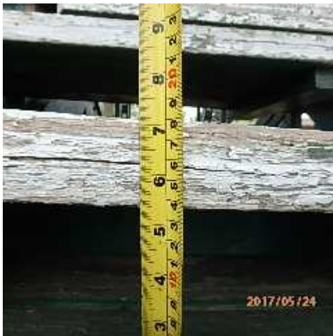
Photo 47: Measured riser height of 7".
