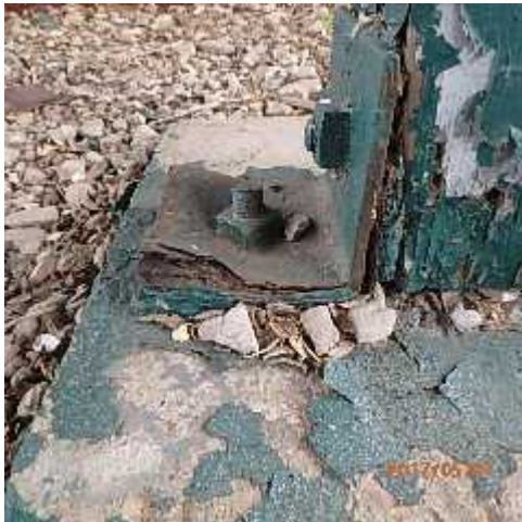
Photo 43: Corrosion of anchor to footing.
