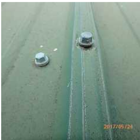
Photo 7: Loose metal roof screws.
