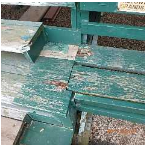
Photo 35: Wood rot at floor boards.
