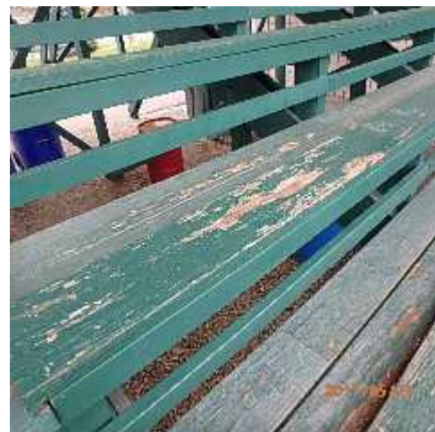
Photo 36: Deterioration of seat boards.
