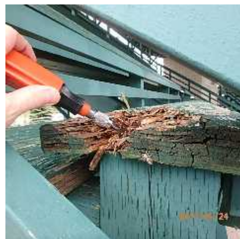
Photo 30: Wood rot at seat board.
