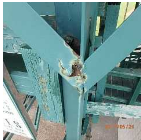
Photo 22: Knee brace corrosion.
