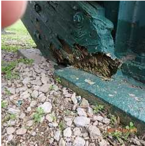
Photo 41: Rotted stringer base.
