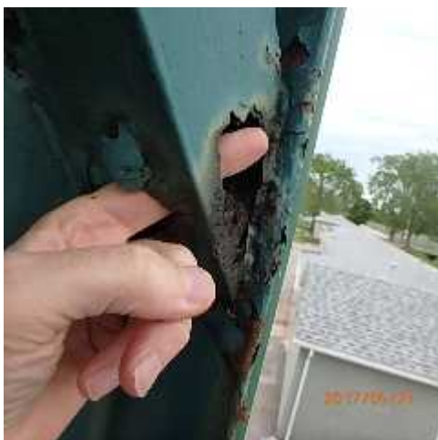
Photo 21: Severe corrosion at water trap.
