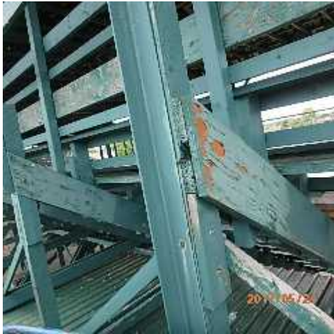
Photo 31: Wood rot at diagonal bracing.
