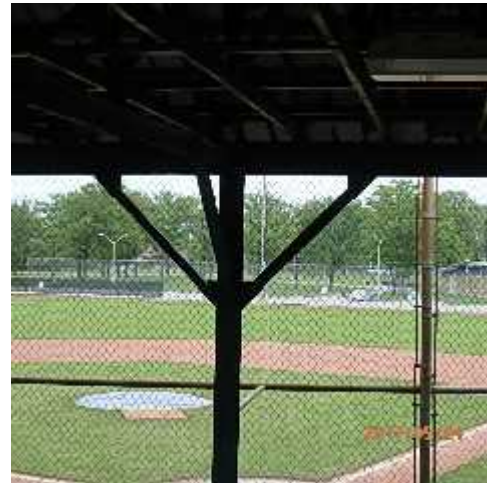
Photo 20: Diagonal knee bracing in vertical planes.
