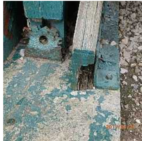
Photo 44: deteriorated post and stringer.
