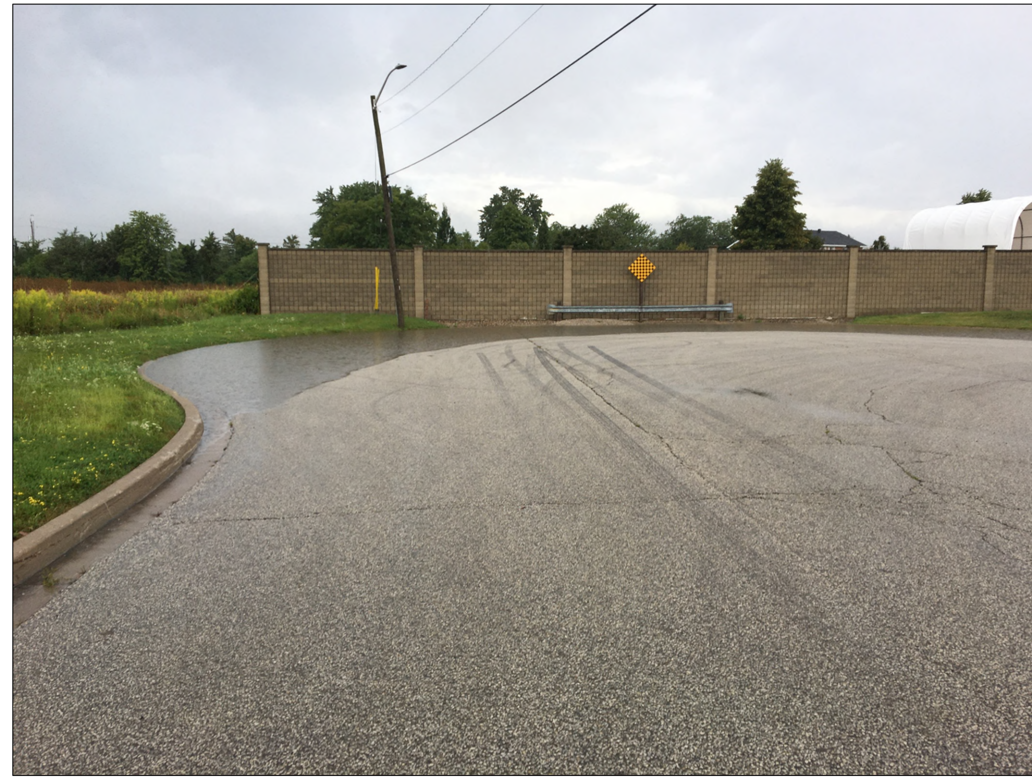
ROSCON INDUSTRIAL DRIVE CUL-DE-SAC (9:56AM) ROADSIDE PONDING – RECOMMEND OVERLAND RELIEF
