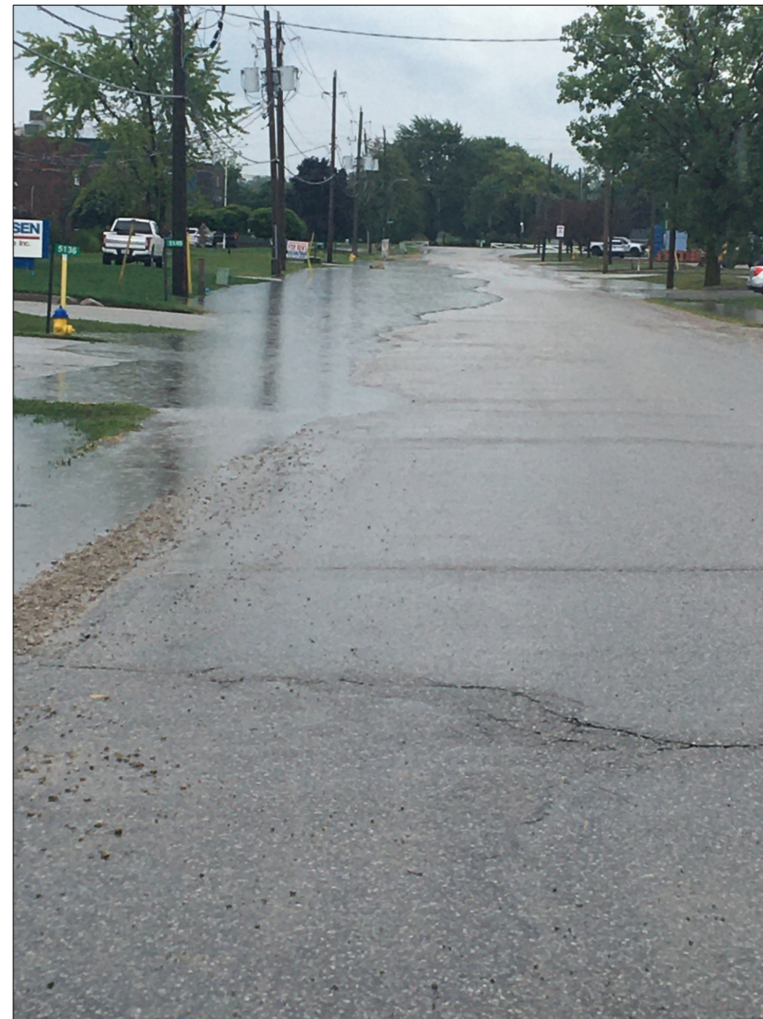
URE STREET (10:16AM) ROADSIDE PONDING – POOR DRAINAGE
