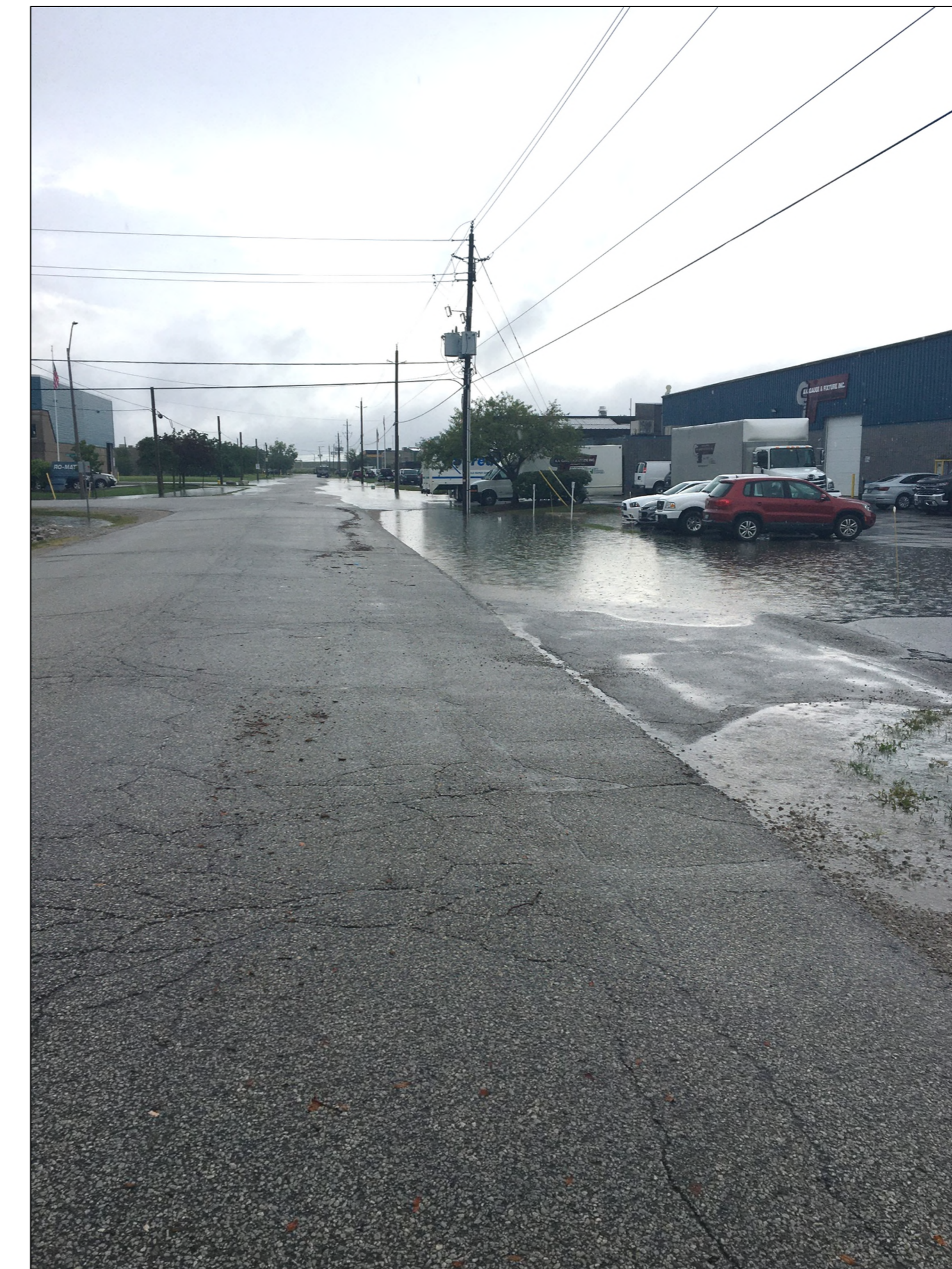
DEL DUCA DRIVE (10:18AM) ROADSIDE PONDING – POOR DRAINAGE
